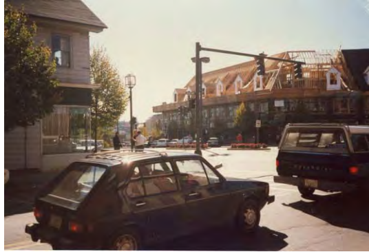
Figure 20: In 1987 the Morrill Block underwent a significant renovation to allow for increased residential units in Dover's downtown. The renovations also increased retail and office opportunities and provided a key to the vibrant location it is today.
