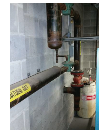
1989 building gas piping
