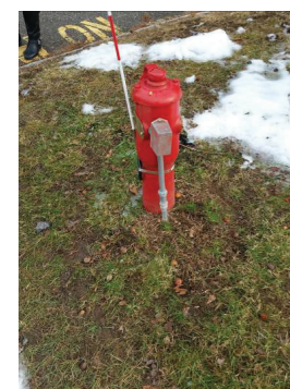
Post indicating valve
