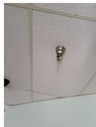
Typical pendant sprinkler
