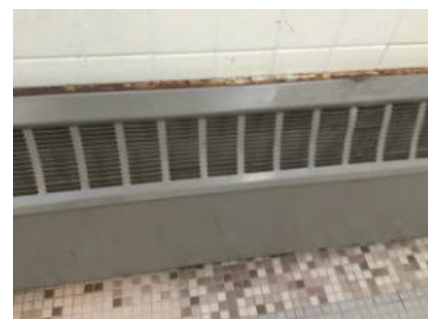
Locker Room Fin tube Radiation
