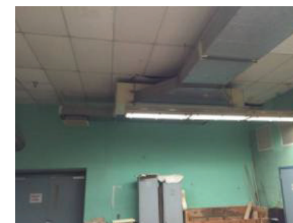
Wood Shop Unit Ventilator
