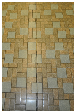
Cracked Tile Floor
