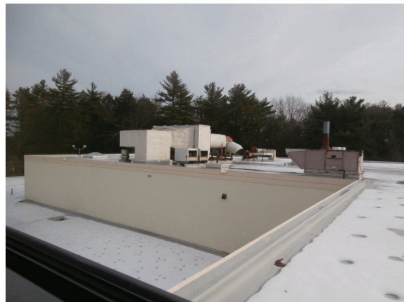
10. High and low roof areas of the 2002 CTC addition, looking NE from the third floor of the 1967 classroom wing.
