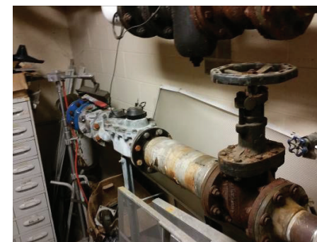
1967 school water service & meter
