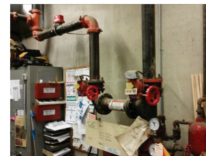
Fire service riser
