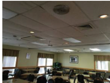
1989 Addition Dining Room - Cassette Type AC Unit (left)
