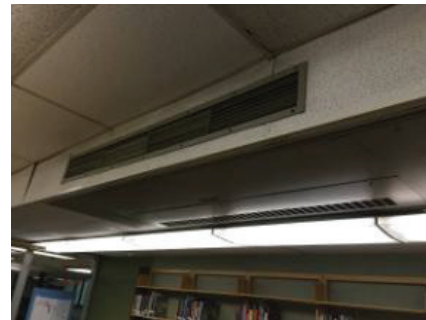
Library Heating & Ventilation Unit
