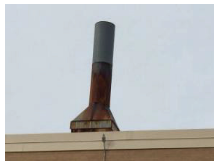
Exterior Boiler Breeching Stack
