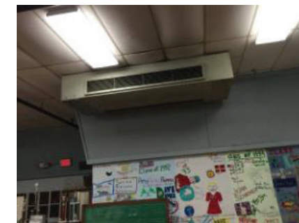
Music Classroom – Unit Ventilator
