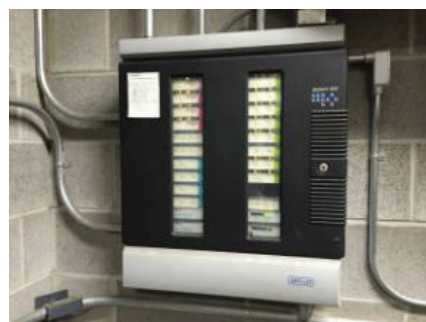
Existing 1989 Addition Building ATC DDC Control Panel
