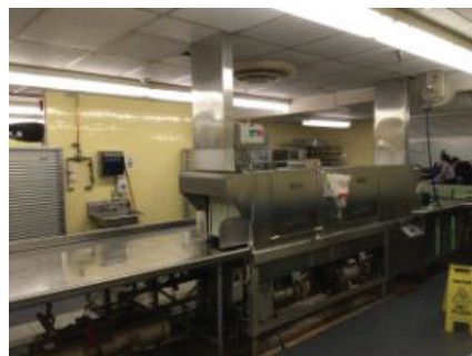
Dishwasher Exhaust Ductwork
