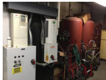
Existing HW Pump VFDs (left) and Expansion Tanks (right)
