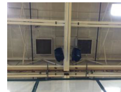
Gym Exhaust Grille
