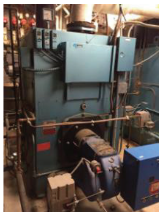
Existing Boiler (Johnson Burner)
