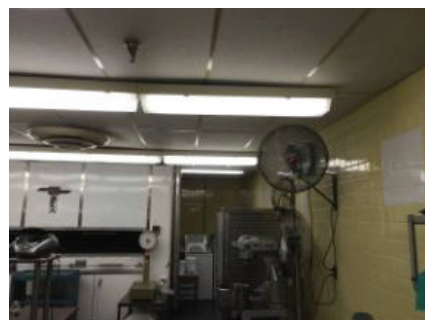
Supply Diffusers (left) and Prop Fan (right)
