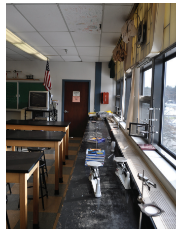
Counter Tops in Disrepair
