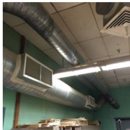
Wood Shop - Ventilation Ductwork
