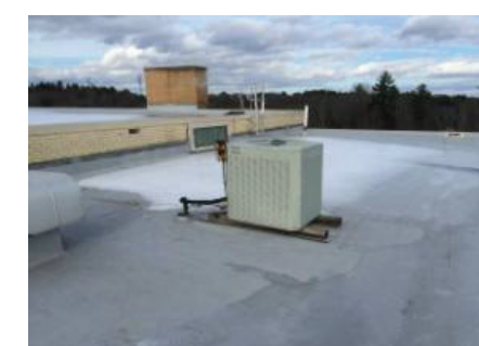
Roof ACC Unit
