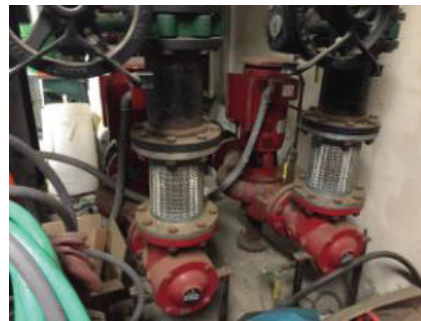
Existing Hot Water Pumps
