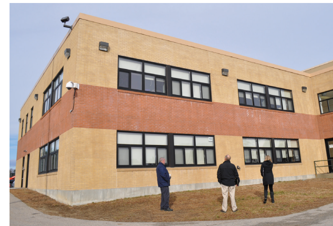
2002 Addition with Visible Efflorescence
