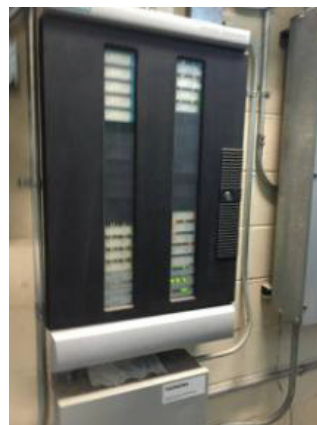
Existing 1967 School Boiler Room ATC DDC Control Panel
