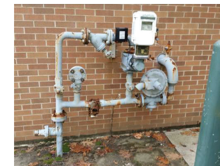
1989 building gas service & meter
