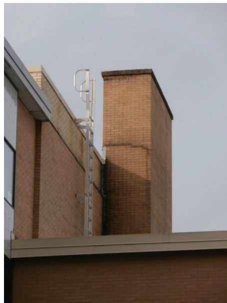
6. Masonry chimney – note step crack near upper roof line.
