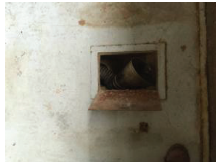
Auto Shop Under Slab Exhaust
