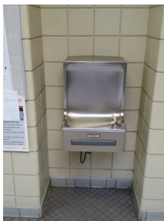
Electric water cooler
