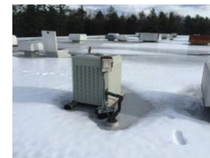
Roof ACC Unit
