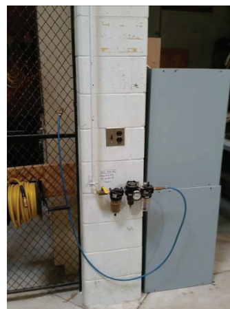
Typical air outlet station
