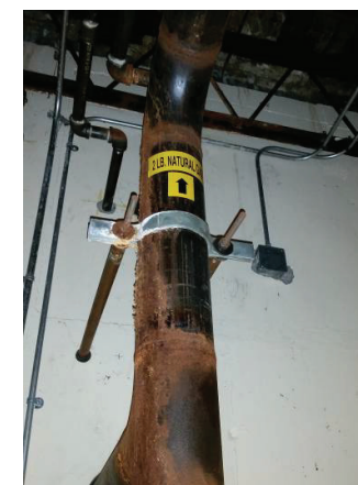
Original building gas piping
