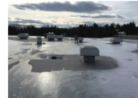
Roof Intake and Exhaust Air Hoods and Fans
