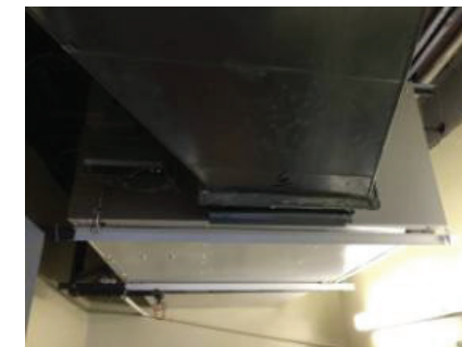
Administration Air Handling Unit
