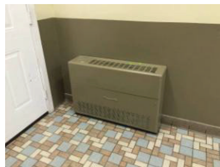
Existing Cabinet Unit Heater
