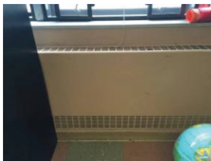
Classroom – Fin tube Radiation
