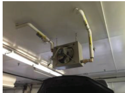
Auto Shop Unit Heater
