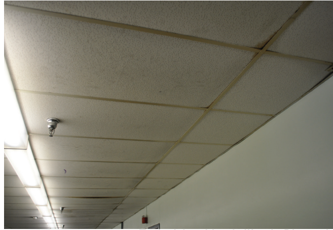
Typical Corridor Ceiling in Disrepair
