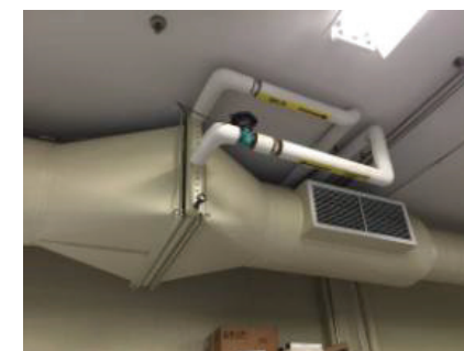
CADD Shop Heating Coil and Ventilation Ductwork
