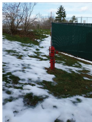
Post Indicating valve
