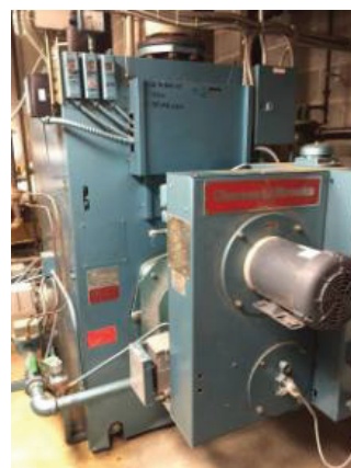
Existing Boiler (CB Burner)
