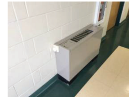
Existing Cabinet Unit Heater – World Arts Wing
