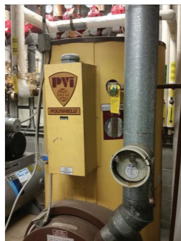
1989 Addition water heater
