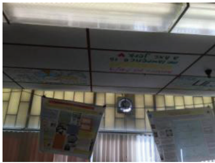
Science Classroom Sidewall Exhaust Fan
