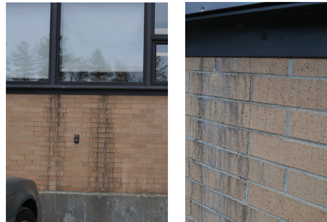
Stained Brick Under Curtain Wall System
