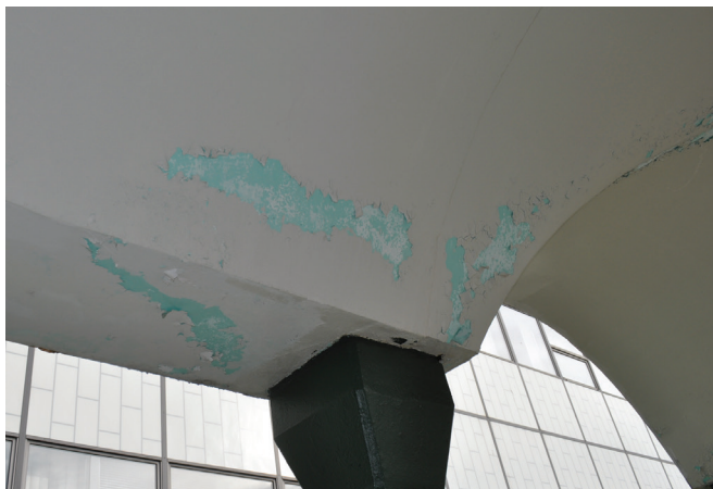
Flaking Plaster at Entrance Canopy
