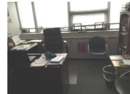
Administration Office – Fin tube Radiation Heating
