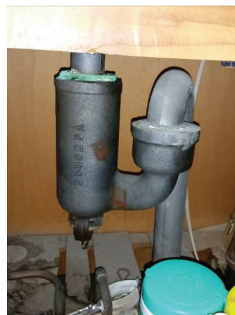
Science waste piping
