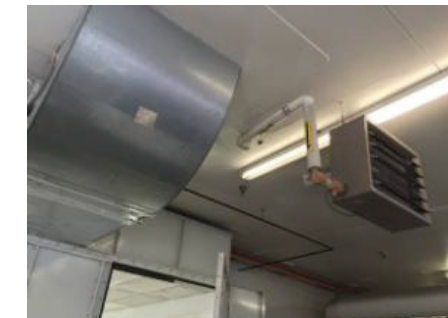
Paint Booth Ductwork and Unit Heater
