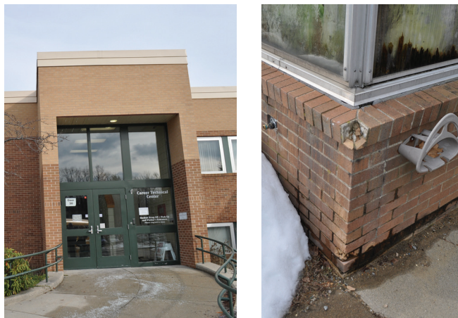
CTC Entrance & Brick in Disrepair
