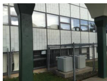
Grade Mounted Air Cooled Condensing Units
