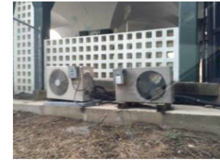
Ductless AC Unit ACC Units
