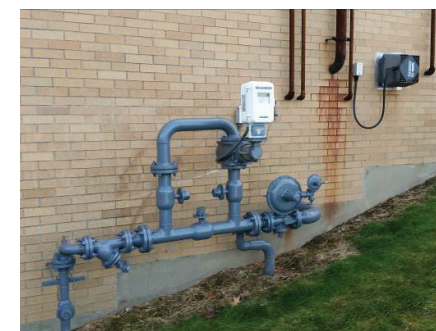
Original building gas service & meter
