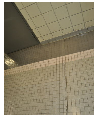
Cracked Tile Floor
