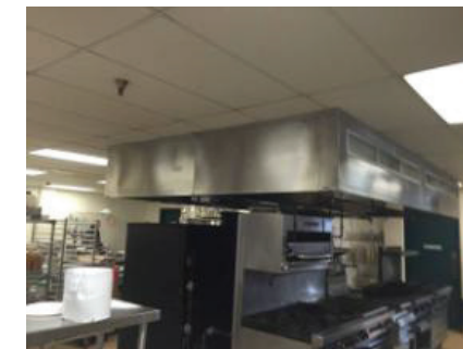
Kitchen Exhaust Hood
