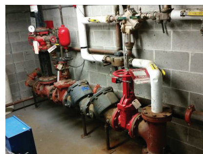
Combined water service - FP riser
