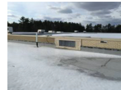
Unit Ventilator Intake Louver
