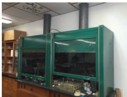
Science Classroom Fume Hoods
