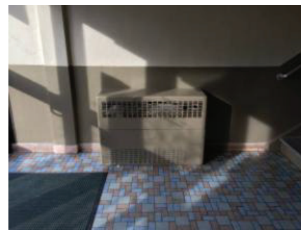
Existing Cabinet Unit Heater
