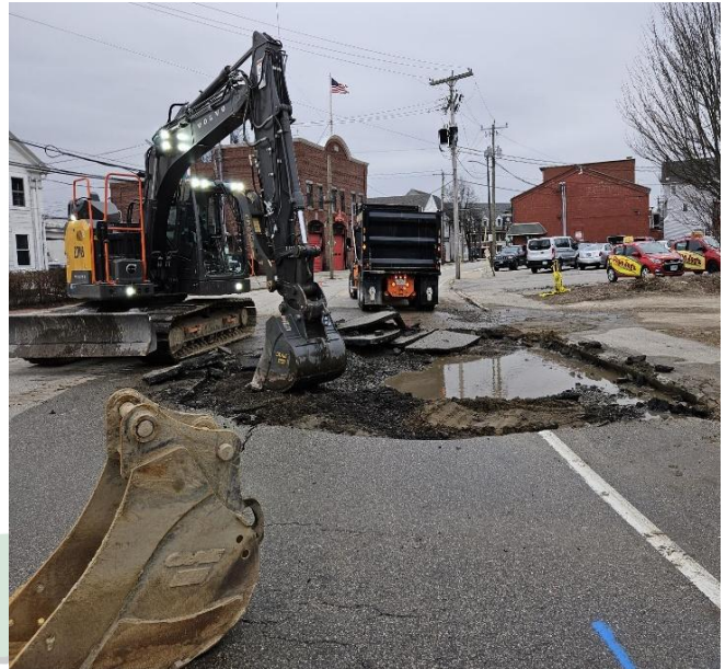
Figure 7: Water main break on Broadway.
