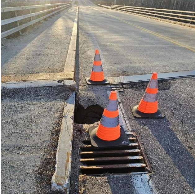
Figure 8: Sink hole on the Fourth Street bridge.
