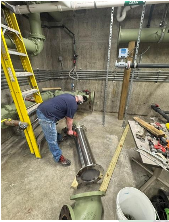
Figure 16: Brand new piping.
