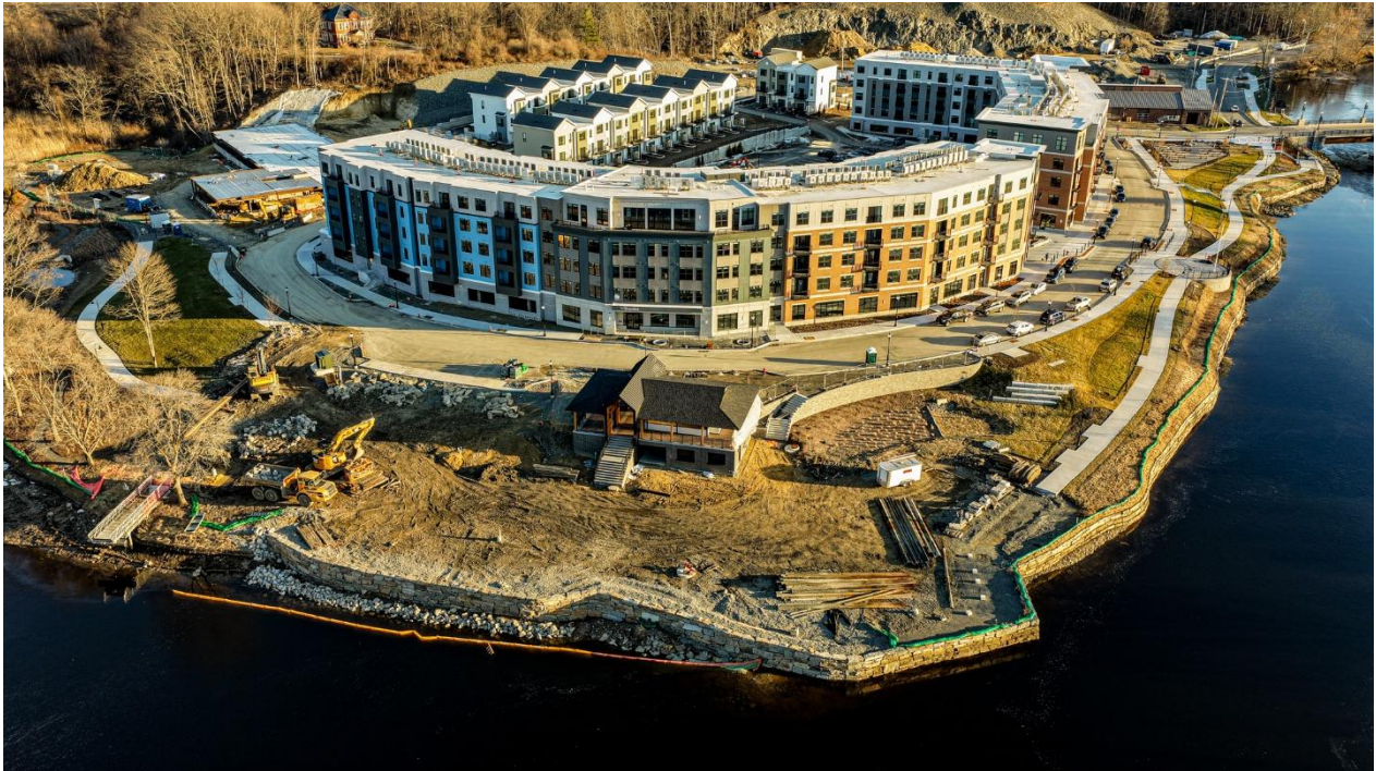
Figure 4: While the completion of the Pavilion is pending due to the temperature sensitivity tasks the crews were able to finish the granite toe wall.
