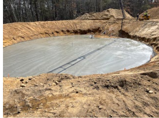
Figure 1: Foundation prep for the new water storage tank on Smith Well Rd.
