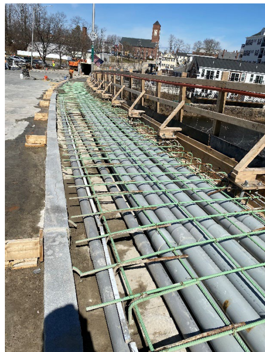
Figure 2: Eastern sidewalk on Chestnut St Bridge with new utility conduit and reinforcing. Sidewalk concrete being poured in the background.
