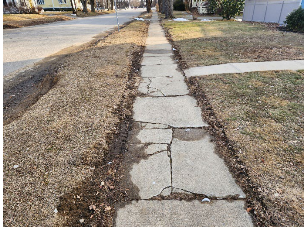
Figure 10: Existing failed concrete sidewalk.
