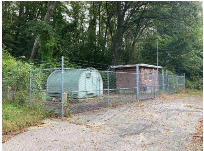
Figure 9: Mill Street Pump Station.
