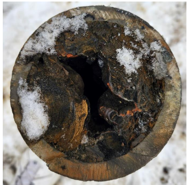
Figure 7: 1880s vintage 4-inch cast iron water main within Angle Street that is being replaced due to repeated failures. The pipe's capacity has been reduced significantly due to build up within the pipe.
