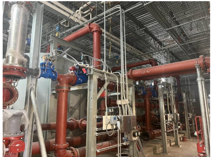
Figure 8: Interior of the new Pudding Hill Water Treatment Plant that treats upwards of 1 MGD of drinking water.
