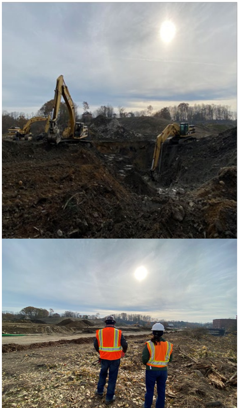
Figure 5: Excavation of the former WWTP Clarifiers (top). Waterfront Construction Manager Jamie Stevens and Assistant City Engineer Jillian Semprini, PE oversee work on the Waterfront.
