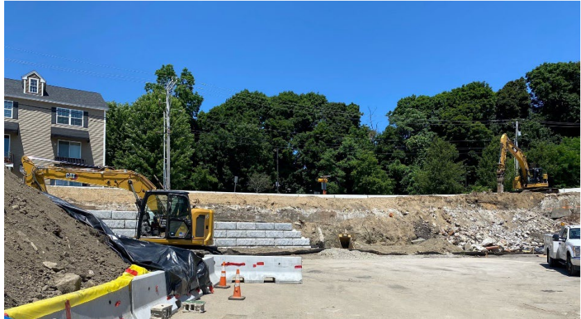
Figure 5: Portland Avenue Retaining Wall is rising.
