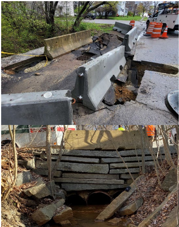
Figure 6: Failed triple culvert below Hough Street.
