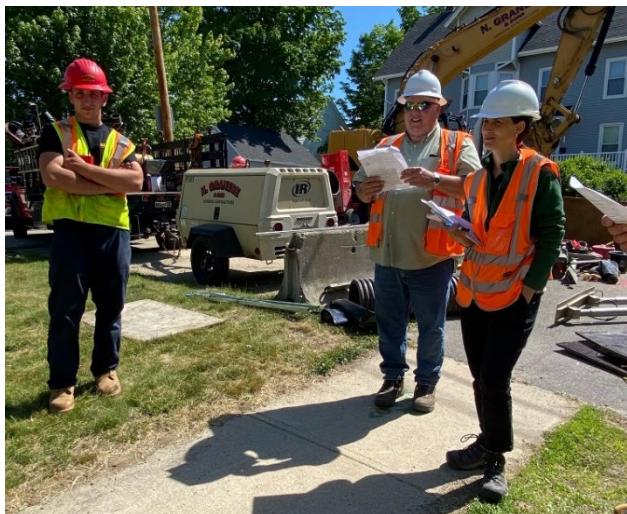
Figure 12: Assistant City Engineer Jillian Semprini and Special Projects Advisor Bill Boulanger meet with the contractor N. Granese and Sons at the corner of Fourth and Fifth Streets.
