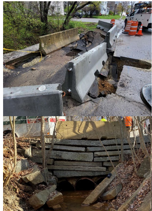
Figure 6: Failed triple culvert below Hough Street.
