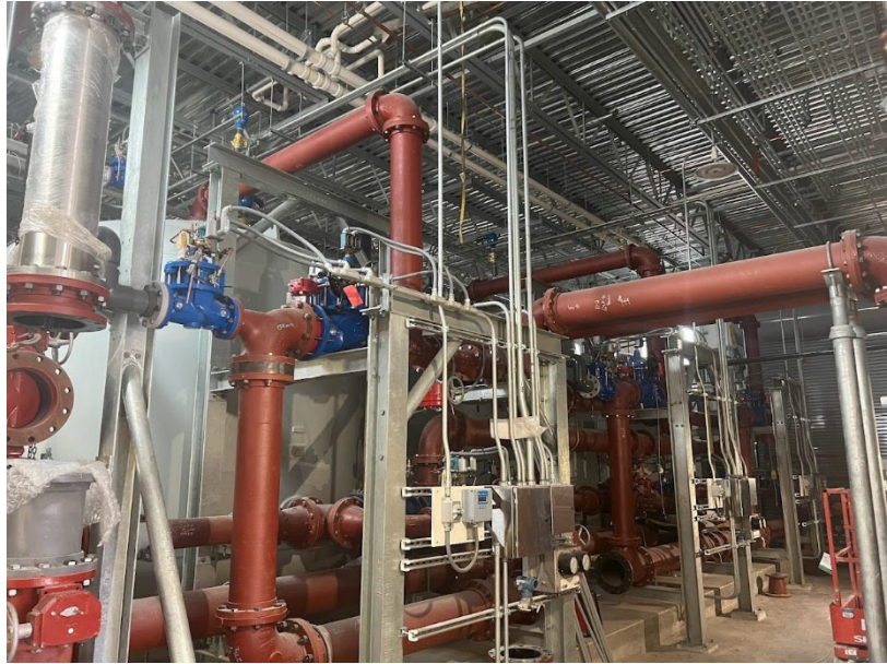
Figure 1: Internal piping and electrical installation continues to progress on the Puttying Hill water Treatment Facility.
