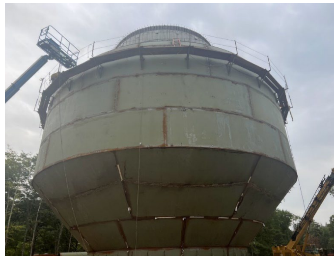
Figure 5: New Tank being welded in preparation for raising to the top of the pedestal.
