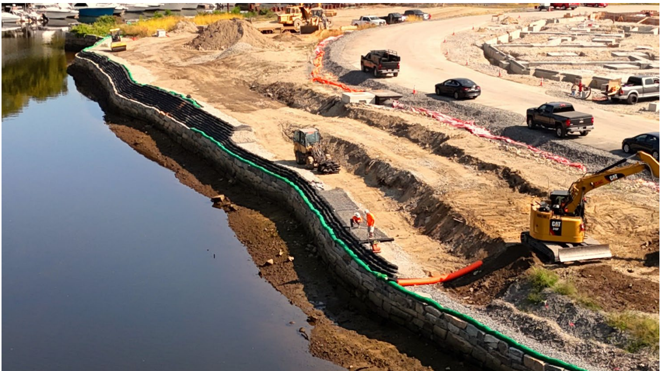
Figure 10: Installation of the flexible mechanically stabilized earth wall (MSE) along the Cochecho River.
