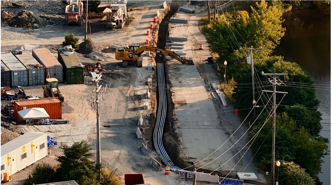
Figure 9: Utility duct bank installation in Payne Street progresses along in preparation for street reconstruction and paving.
