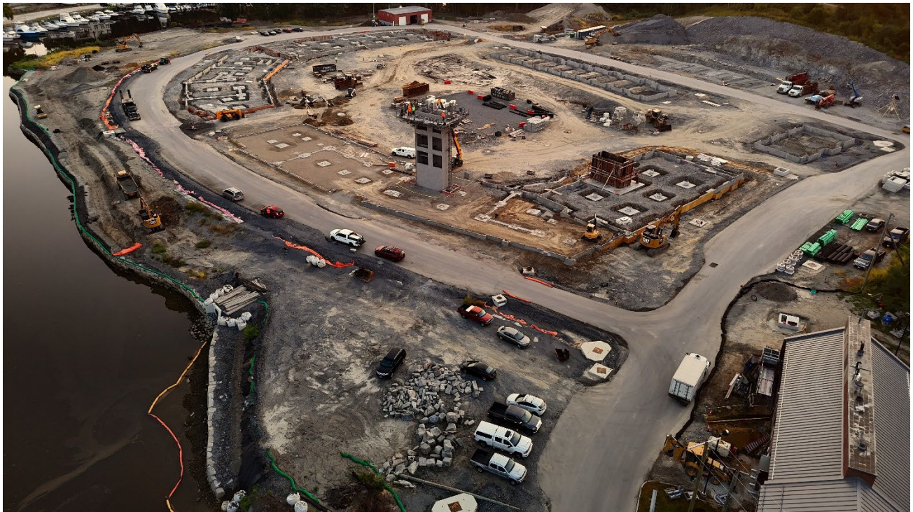
Figure 8: Foundation work on the private development continues with the construction of the elevator shafts.
