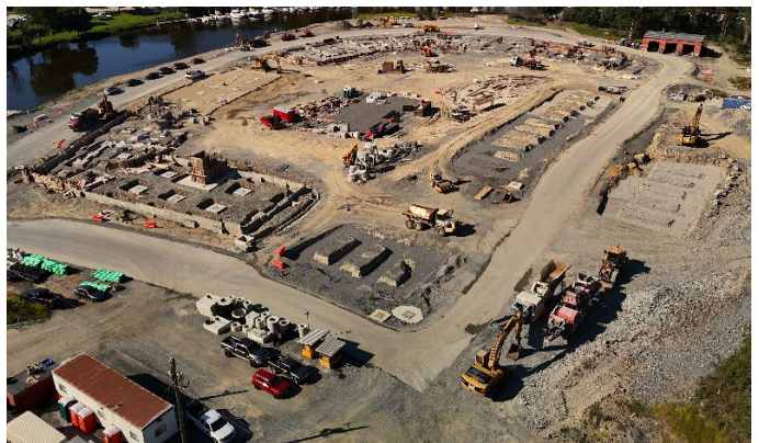
Figure 7: Foundation work for the private development continues to prepare for vertical construction.
