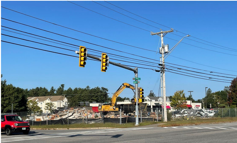
Figure 10: Demolition of the R&W Building on Central Ave to prepare for the new Chase Bank.
