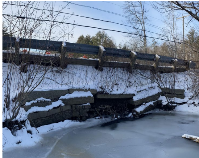
Figure 15: Upstream Entrance to the failed County Farm Road Culvert
