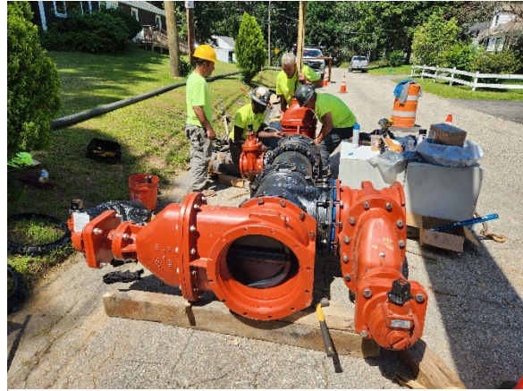
Figure 6: New valve assembly was installed in Glenwood Ave for the new water main in Smith Well Road.
