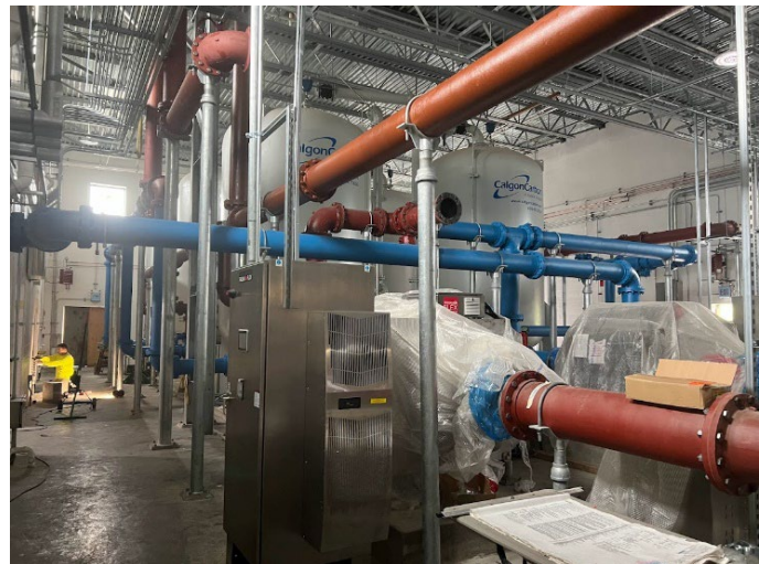
Figure 2: Interior fit up continues at the new Pudding Hill Water Treatment Plant.
