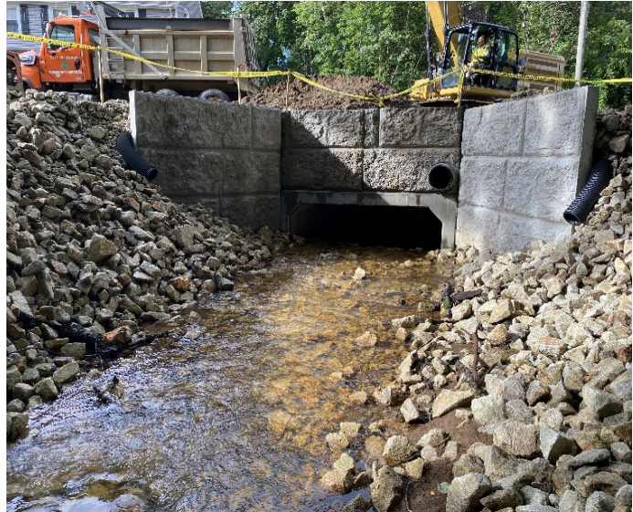
Figure 1: Newly installed precast concrete box culvert below Hough Street. Crews above the culvert are reconstructing the road in preparation of paving.
