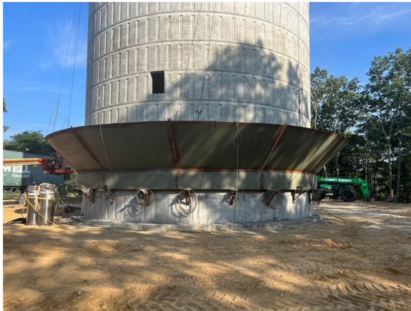
Figure 7: New Smith Well Rd tank fabrication starting at the base of the completed pedestal.
